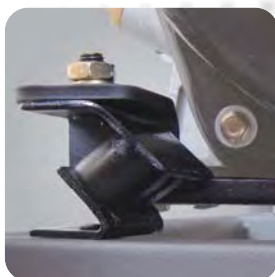
vibration absorber support the whole generator set
